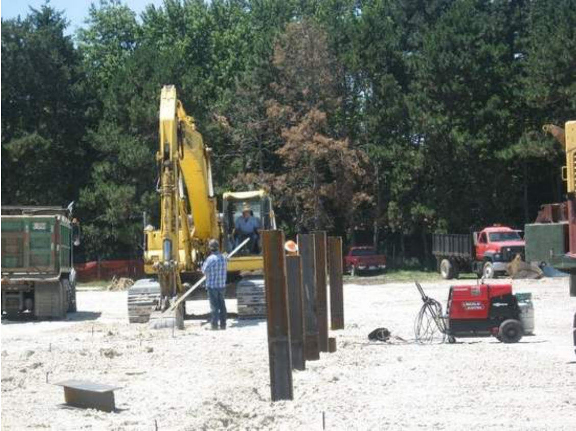
Construction has begun at the site of the new Fremont Middle School. (Dusty Zeitz | News-Messenger correspondent)
