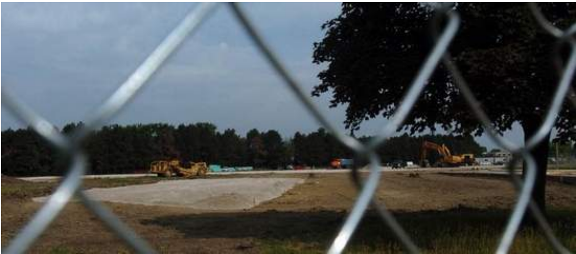
Heavy equipment is seen through a fence June 23 as crews prepare the area next to the Fremont Ross High School for construction of the new middle school. (Jonathon Bird | News-Messenger)
