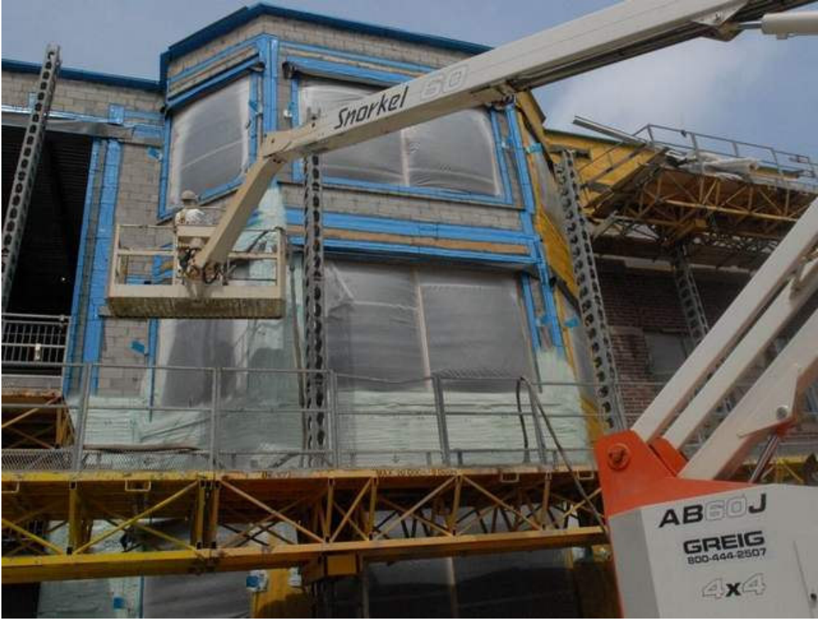
A worker sprays an energy saving foam insulation April 18 on the outside wall of the new middle school in Fremont. / Jonathon Bird/News-Messenger
