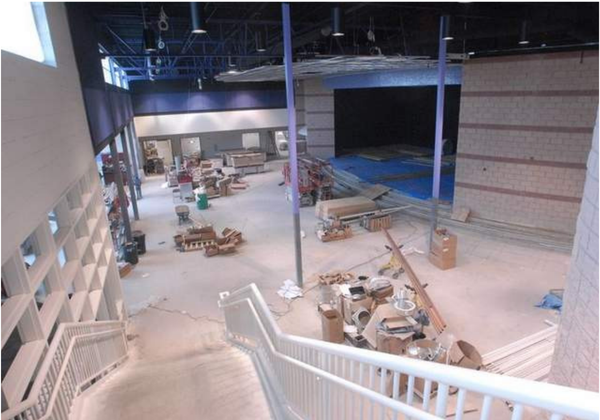
Various supplies and construction equipment sit in the cafeteria of the new Fremont Middle School on Tuesday. / Jonathon Bird/News-Messenger
