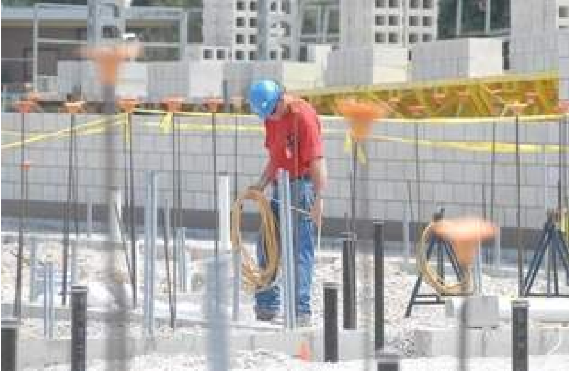
Work continues on the grounds of the new Fremont Middle School. (Jonathon Bird | News-Messenger)
